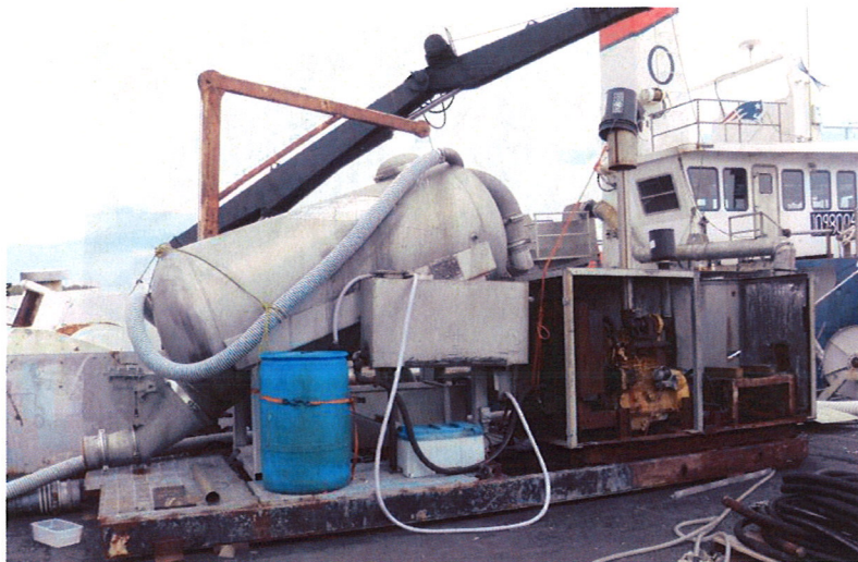
Figure 10. This pump, situated on a dock, is used to move the herring from the boat and into the dewatering box and eventually a truck or container, situated portside.
