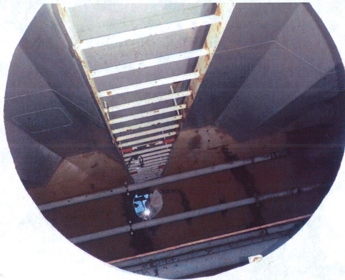
Figure 8. A holding tank, empty
